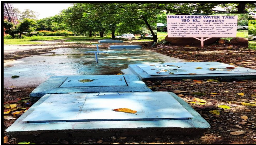
Figure 3.3. Underground water tank of 150 KL capacity
