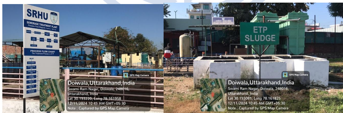
Sewage Treatment Plant and Effluent Treatment Plant (ETP) at SRHU
