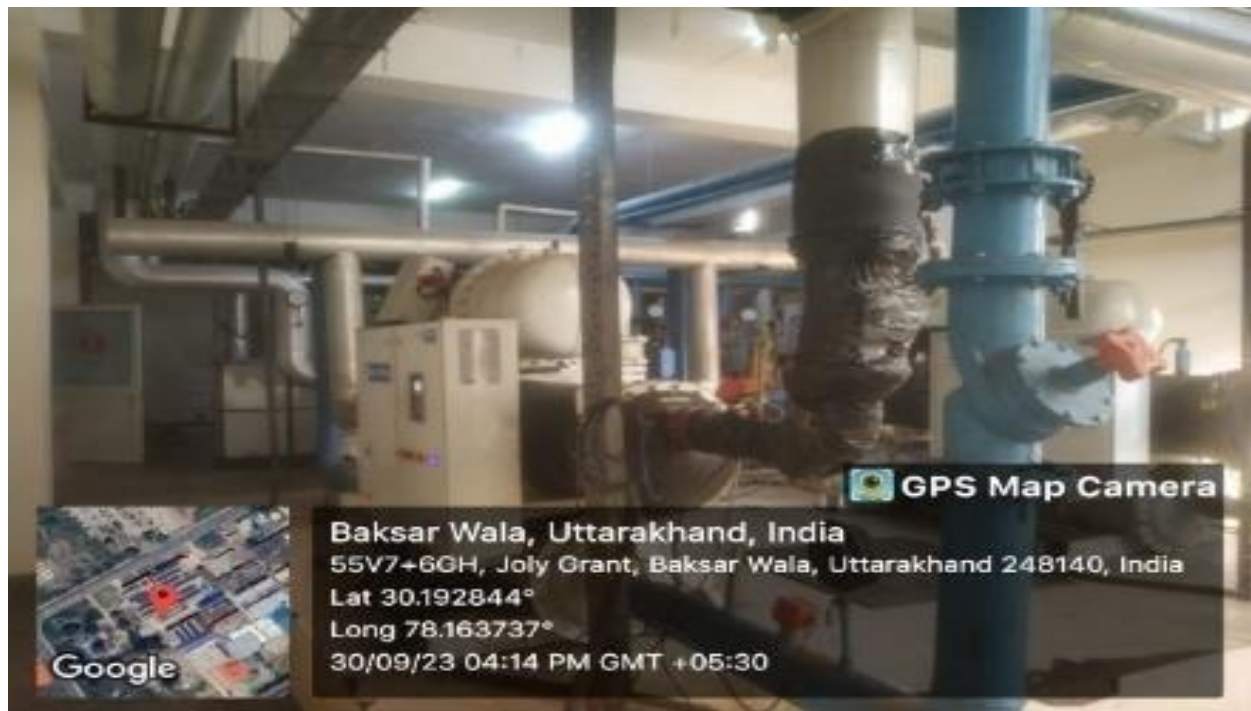
Current HVAC system installed in the university
