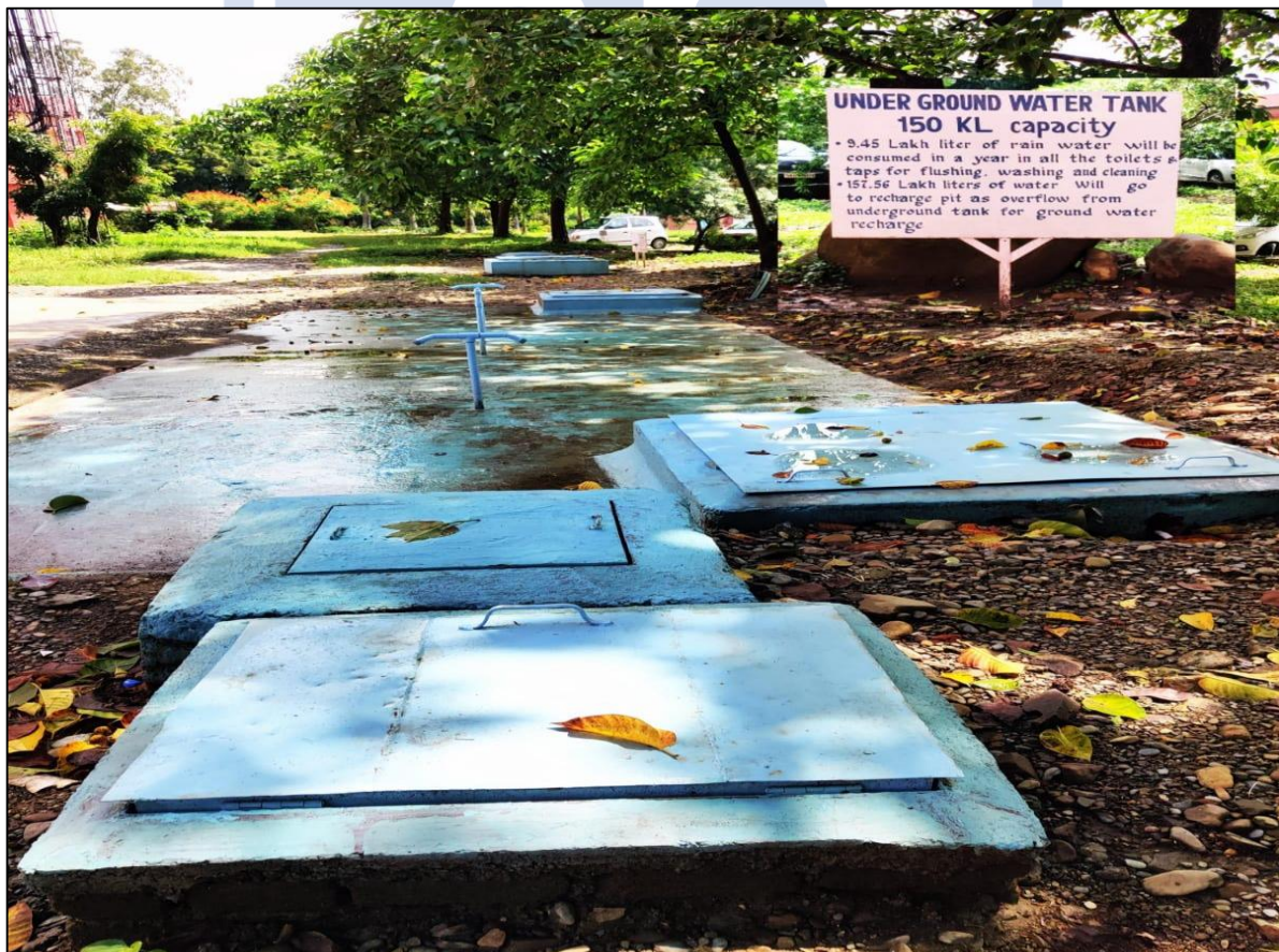
Rain Water Harvesting Tank (capacity 150 KL)
