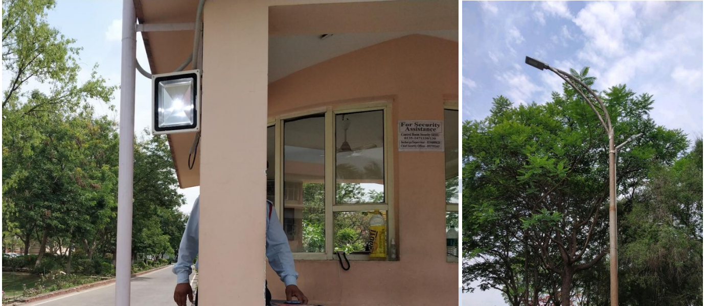
LED lights at security post, near Medical College and the university premises
