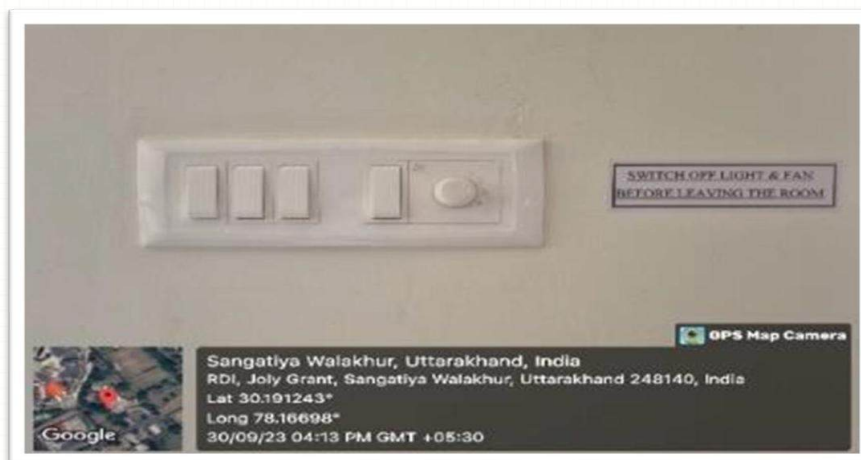
To instil responsible consumption message slips are placed near switches as reminder of user's responsibility
