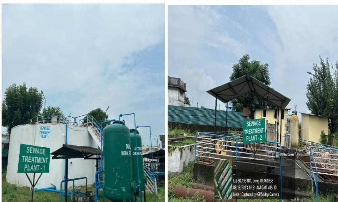
Sewage Treatment Plant no. 1 & 2
