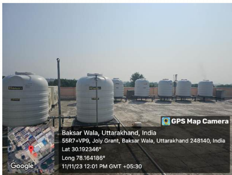
Water tanks on the roof of Trauma Centre Building
