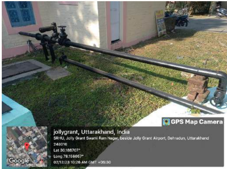
Tubewell no. 3 and water distribution system
