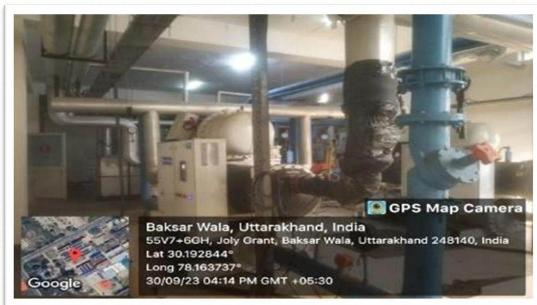
Energy efficient VFD driven pumps in central air conditioning
