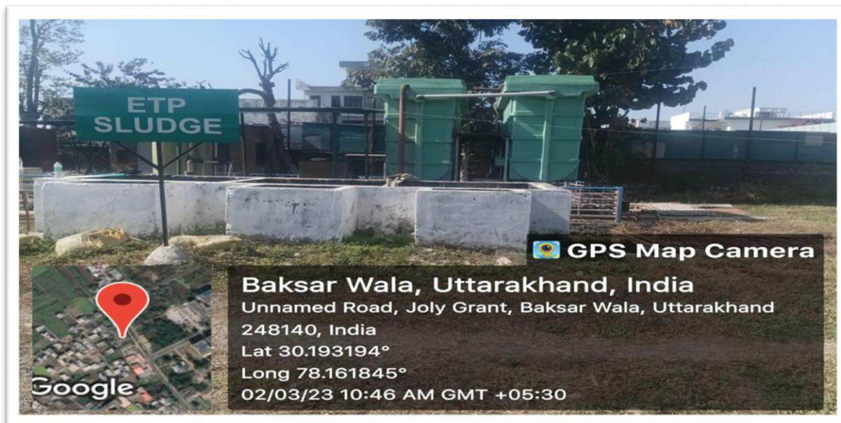
ETP p located at SRHU with an aim to treat effluent promoting sustainable environmental conservation
