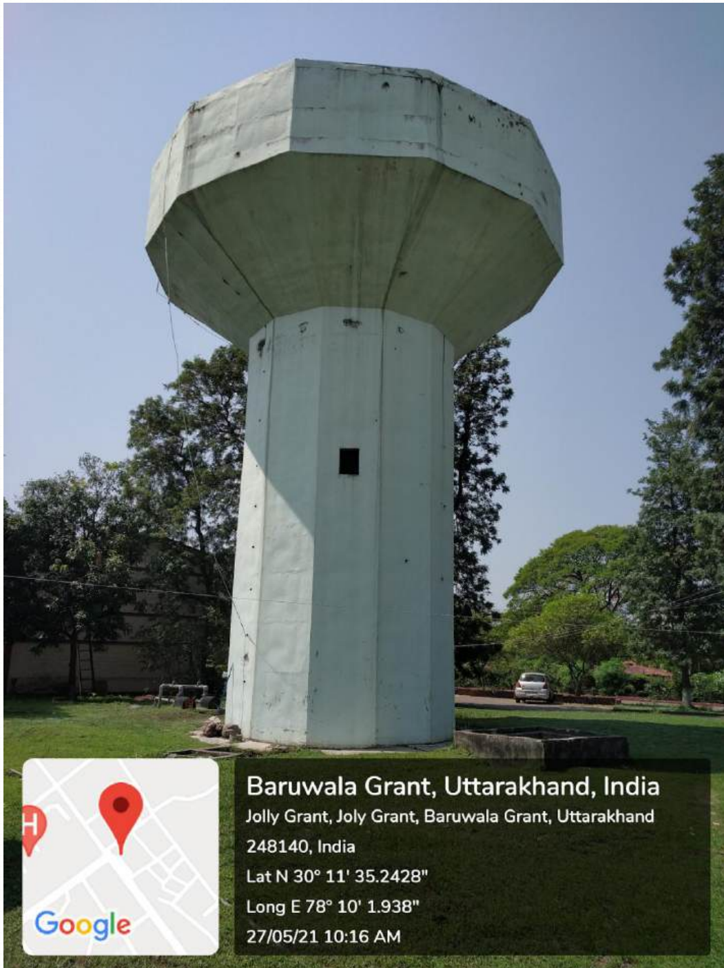
Overhead Tank (Tubewell Chowk) with capacity of 250 KL
