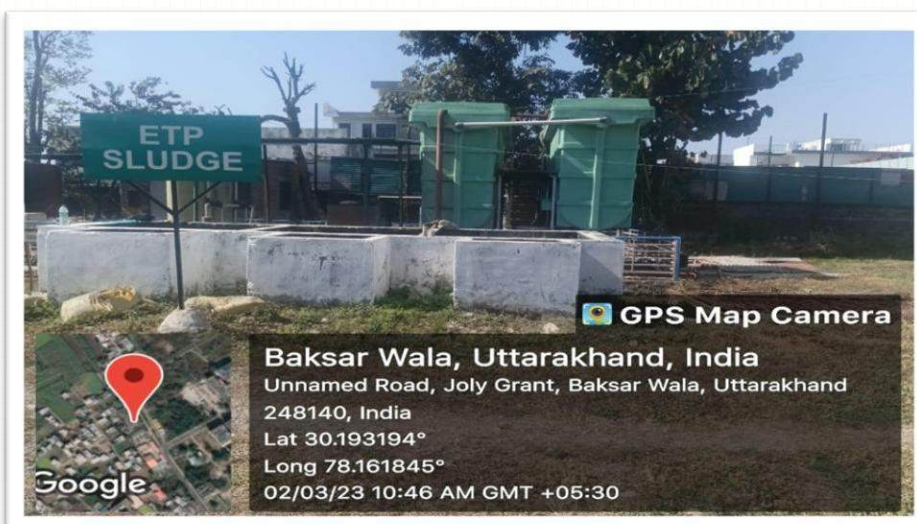
Effluent treatment Plant at SRHU
