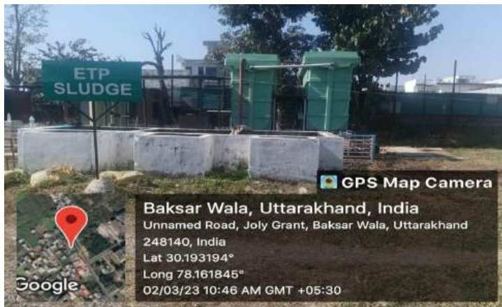
Effluent Treatment Plant (Capacity: 90 KLD)
