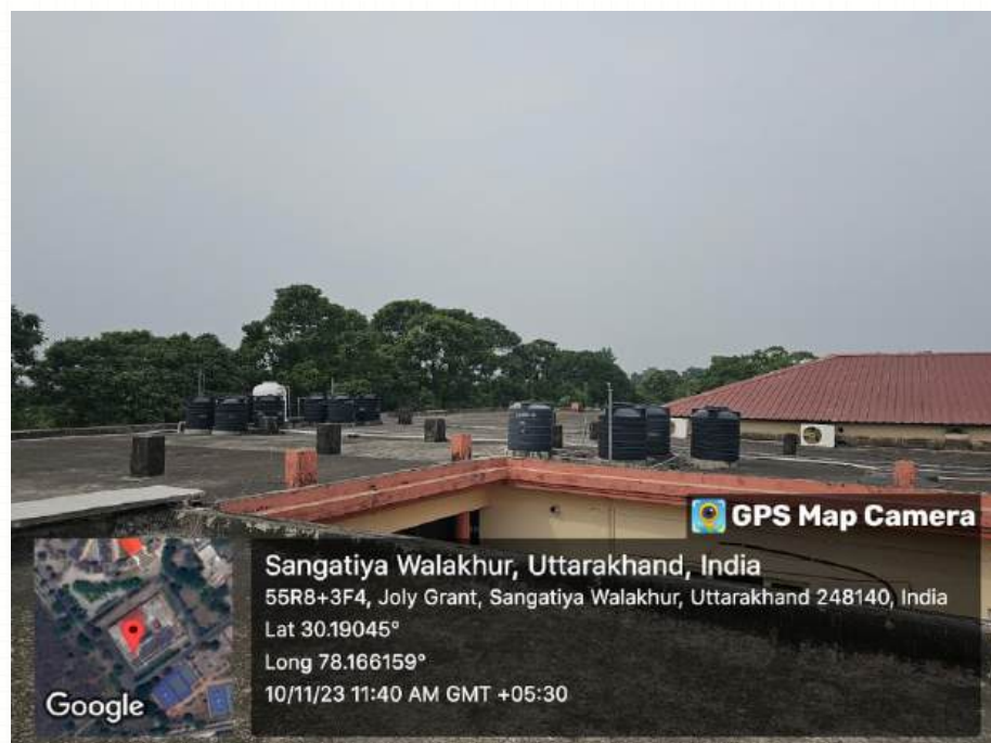
Water tanks on the roof of Nursing College Building
