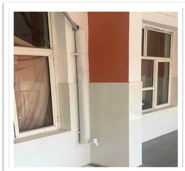
Condensed water collection provision which can be utilized for cleaning purposes
