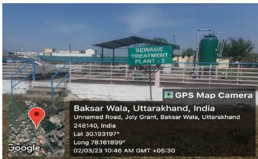
Sewage Treatment Plant with capacity of 1MLD
