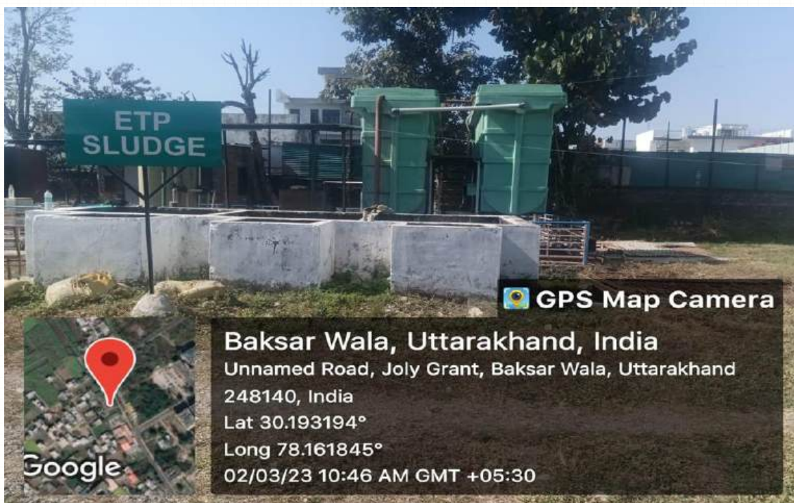
Effluent Treatment Plant (Capacity: 90 KLD) for liquid waste management
