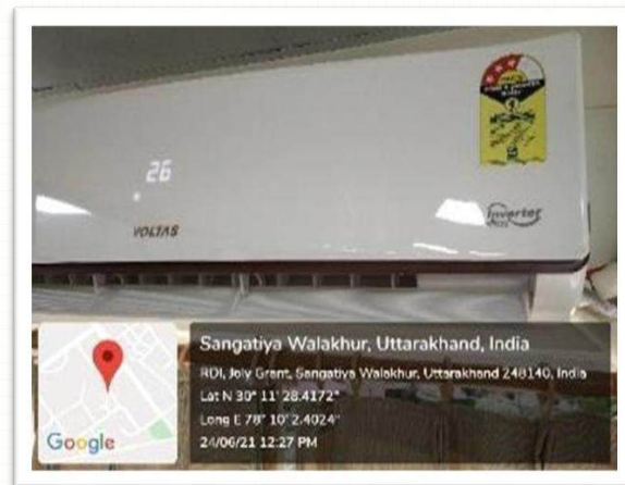
Energy efficient BEE star rated ACs installed at various key locations
