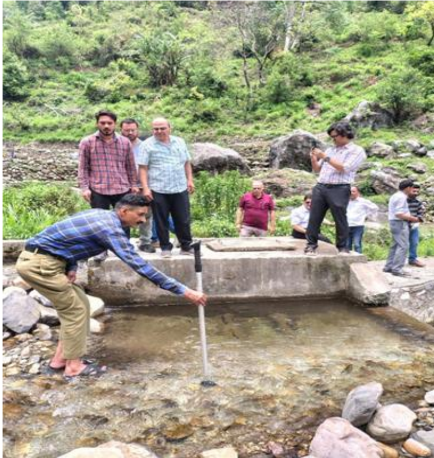
Water being collected post installation of low cost underground water filtration
