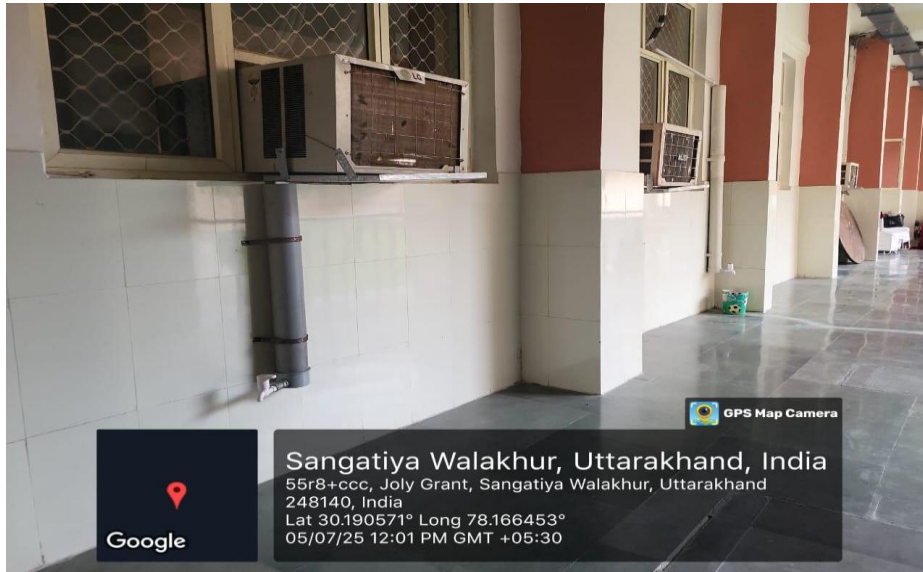
Condensed water from AC Units is used across the campus to repurpose and recycle water
